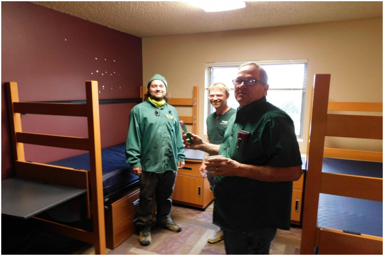
Brandon Hopper-Barraza and Ben Blumstein are servicing HVAC units, while Scott Ellis is patching and painting walls
