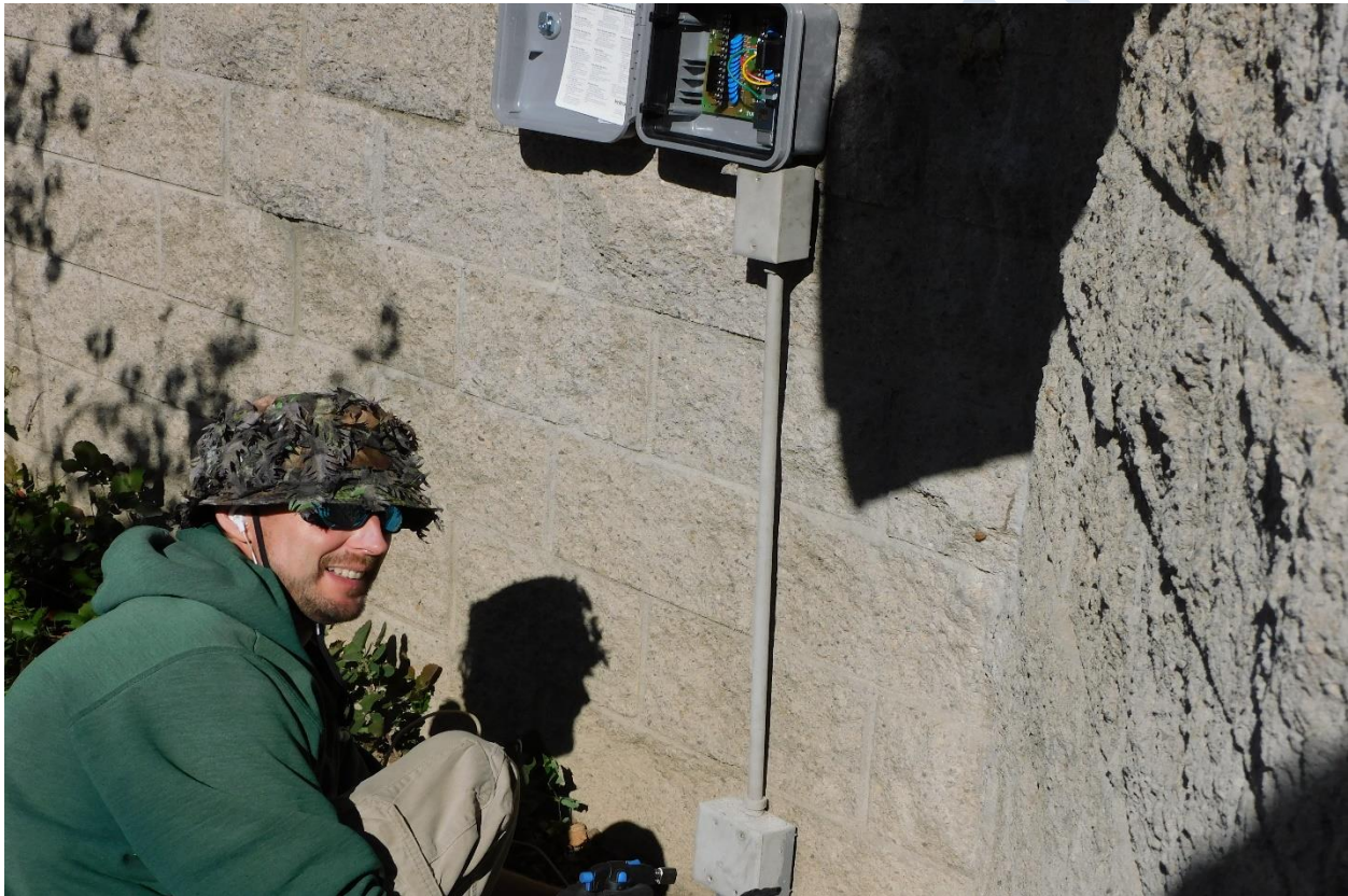
Lead Grounds Technician Sam Johnson repairing the sprinkler controller at the PAC
