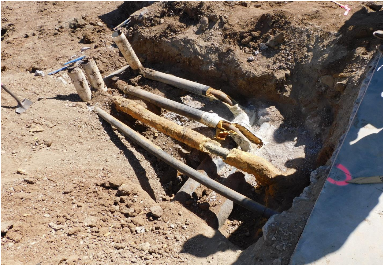
One of the "conflicts" between footer location and existing utilities
