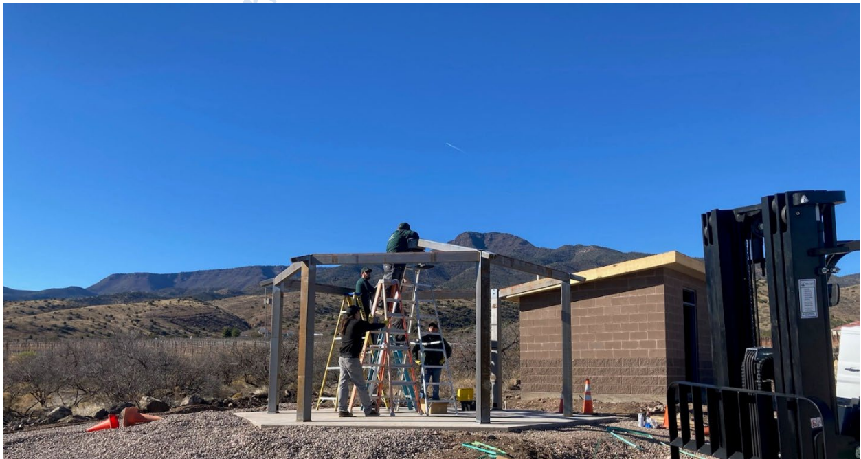
Grounds team members Jonathon Krusze, Brett Rockow, Steve Korniat, and Steve Soto are constructing the new gazebo at the Verde Valley Campus RV Park
