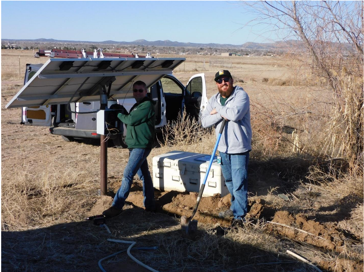
Zack Vannoy and Tim Peterson repair solar electric service to the irrigation pond pump at Chino
