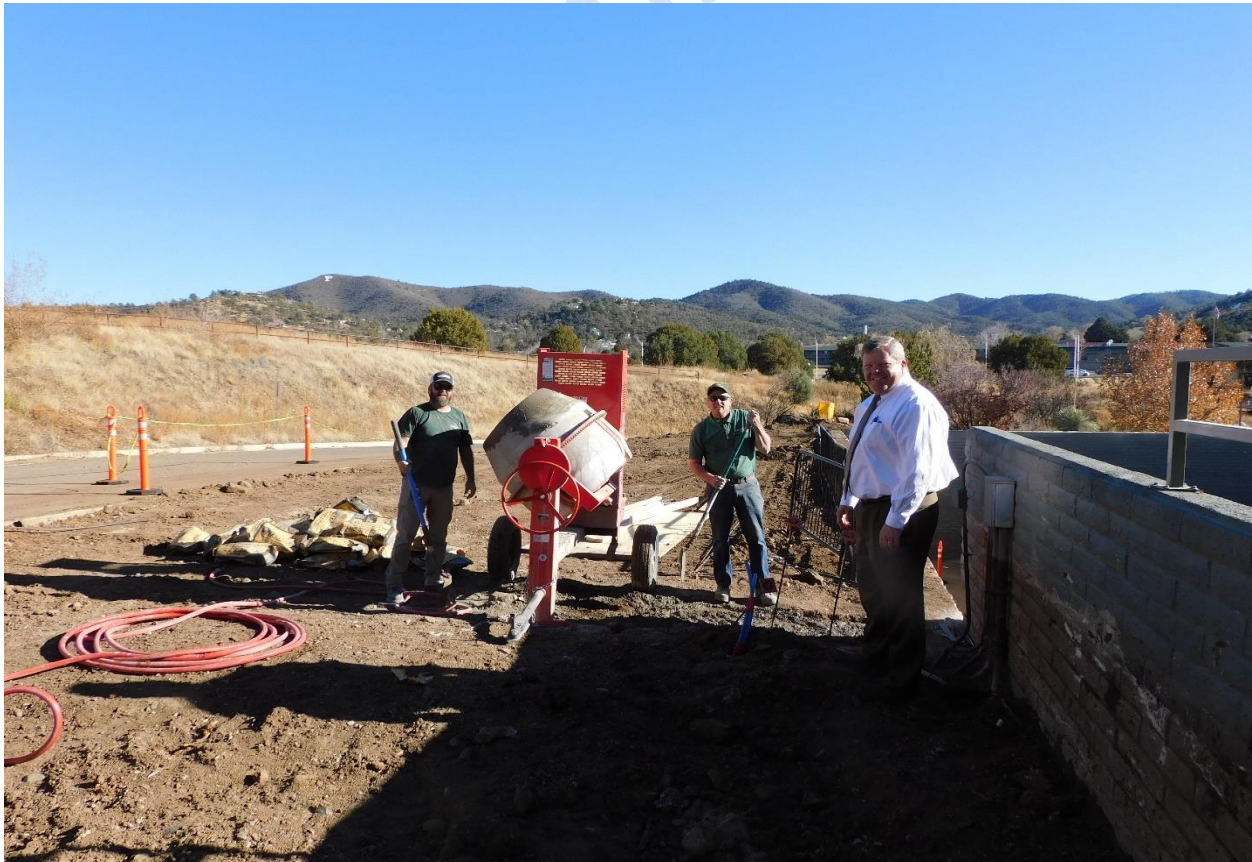
Building 4 retaining wall replacement – Dean Farnsworth’s dream job for the day working with Travis Whorton and Scott Ellis mixing concrete
