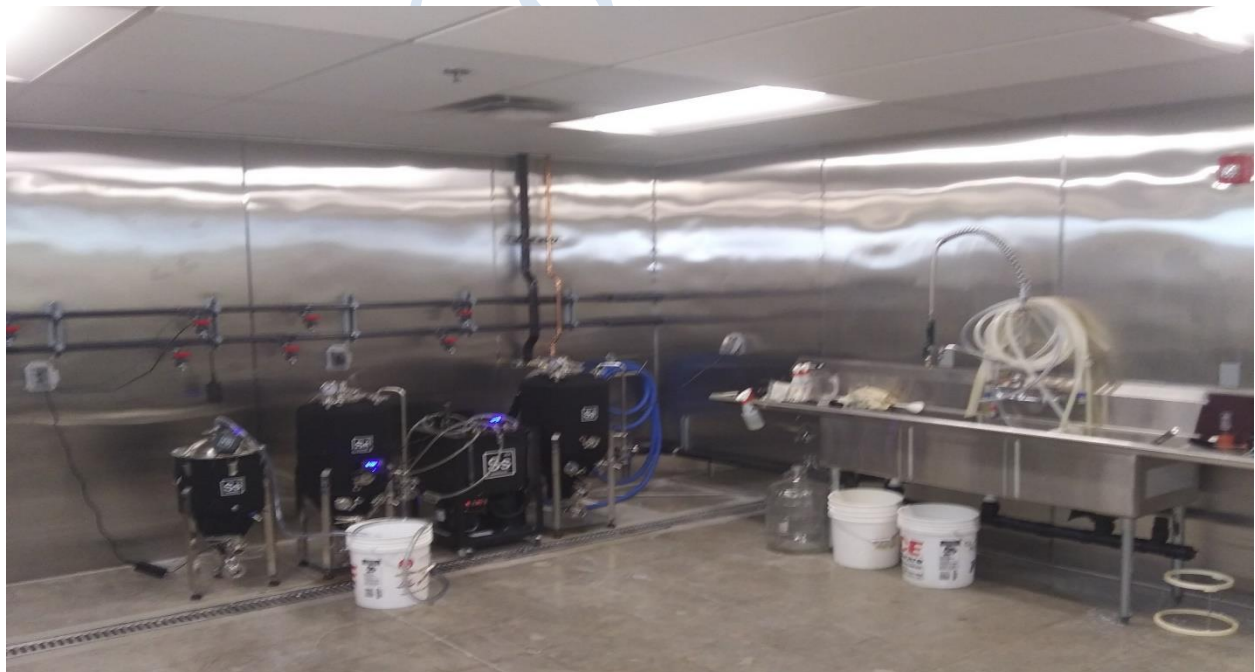
Polished floor and new stainless steel wall treatment and sinks for Brewing
