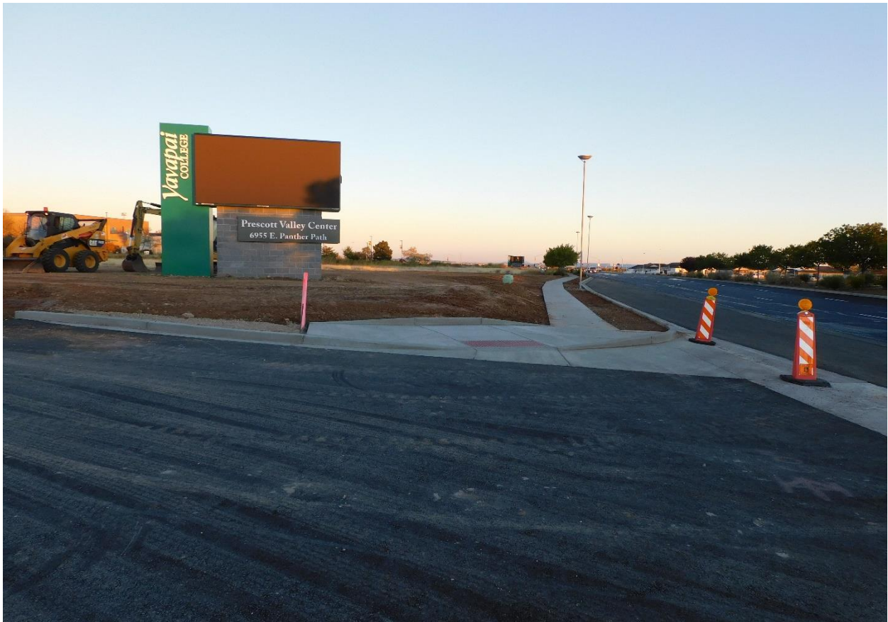
Location of deceleration lane from Glassford Hill Road to the Prescott Valley Center
