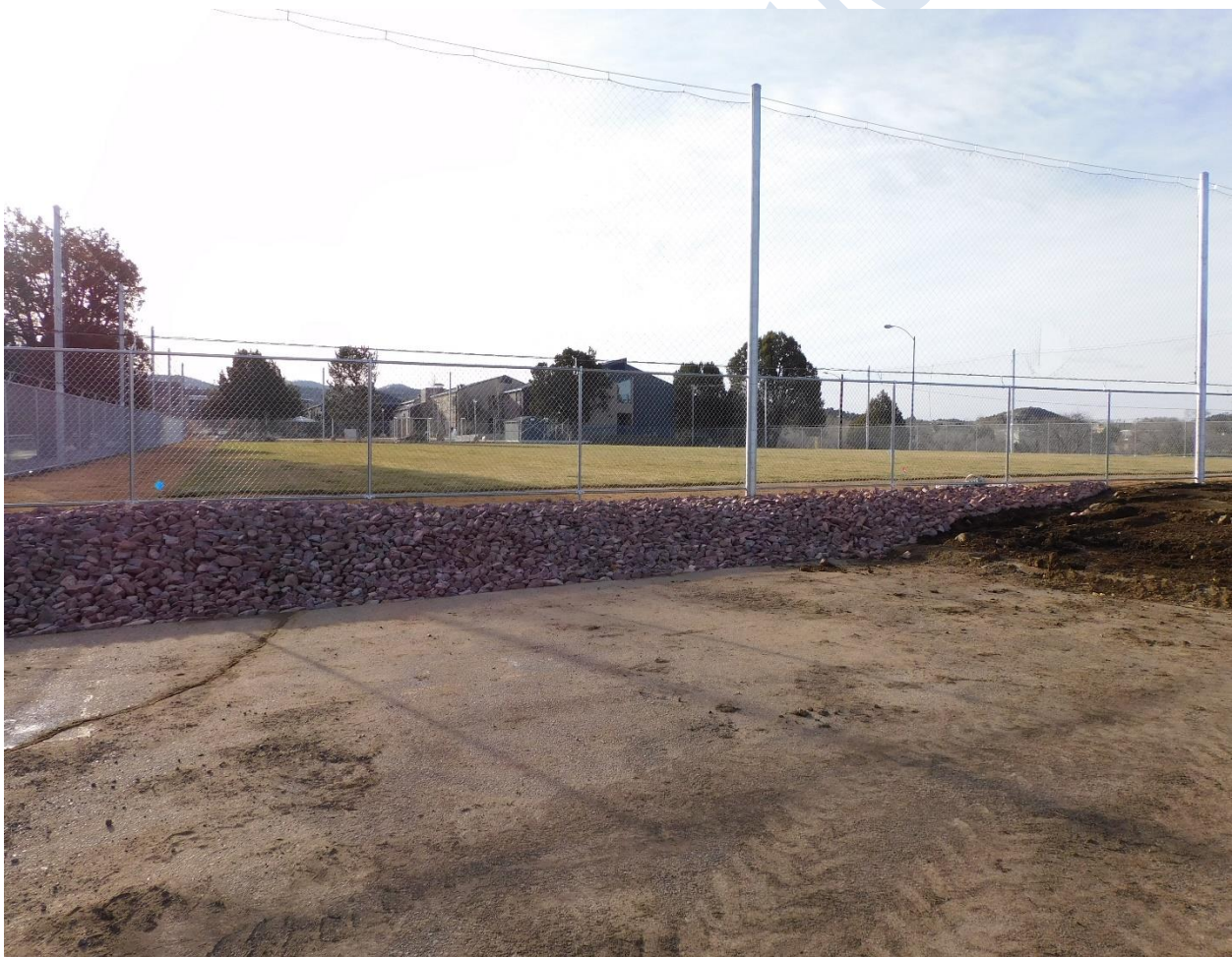
Riprap along the perimeter of the field
